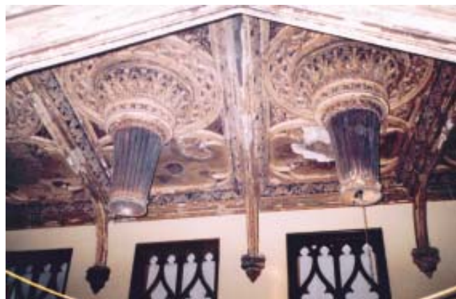
The Crown & Kettle ceiling, fire-damaged but still impressive.
